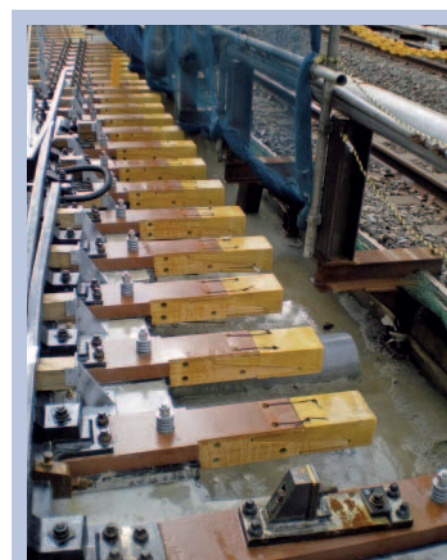
Fig 5: FFU in slab track, switch prepared to install second part later on – SEKISUI
